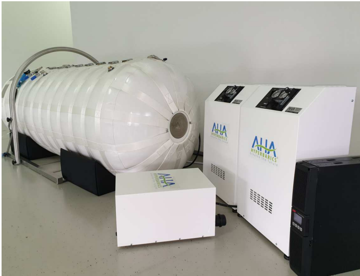
UPS system (positioned on the right side of the picture)
